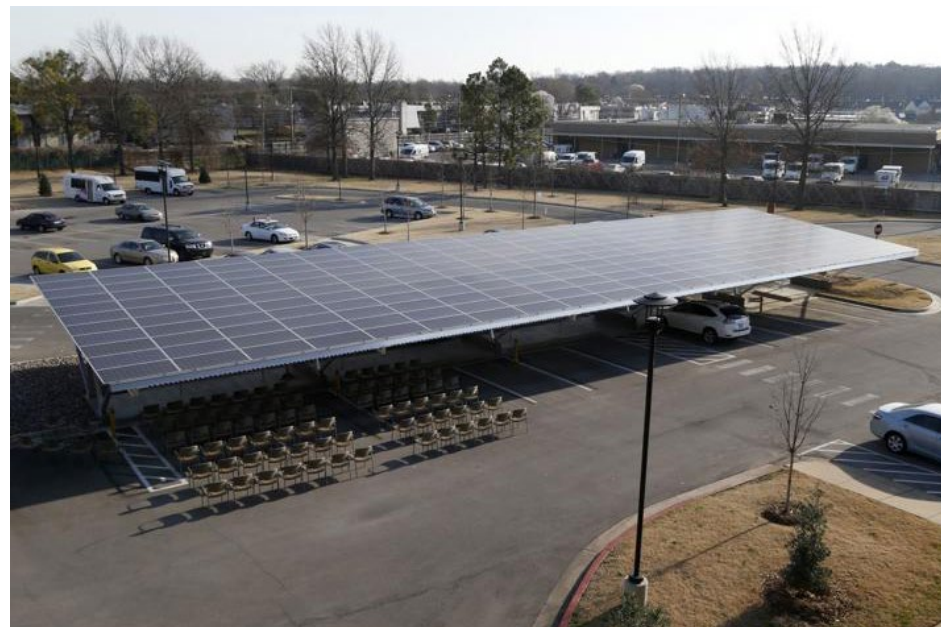
In 2014, Zarrow Pointe installed the first solar parking canopy in Tulsa.
